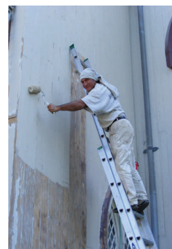
There's always some task to do to maintain one of our lovely older buildings. Here, an exterior wall is painted a few years ago.
